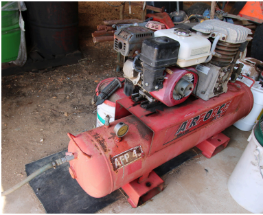
Air Compressor Air Compressor
