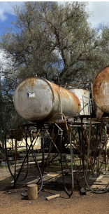
Gravity Overhead Diesel Tank 2
