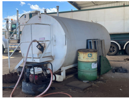
Ashmore Engineering Diesel Tank
